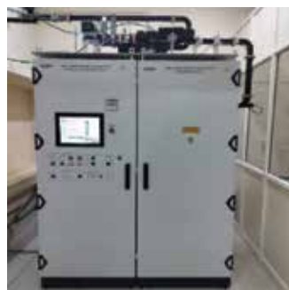
C-Band Radar Transmitter
