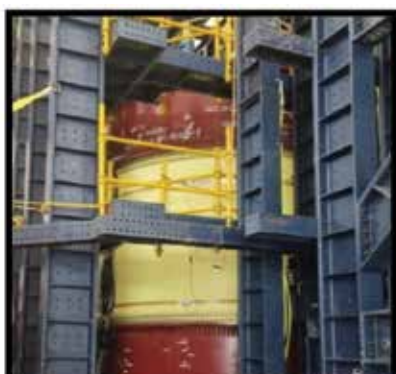
Structural Acceptance Test of Isrosene propellant tank envisaged to be used in SC120 stage for Flight Demonstration
