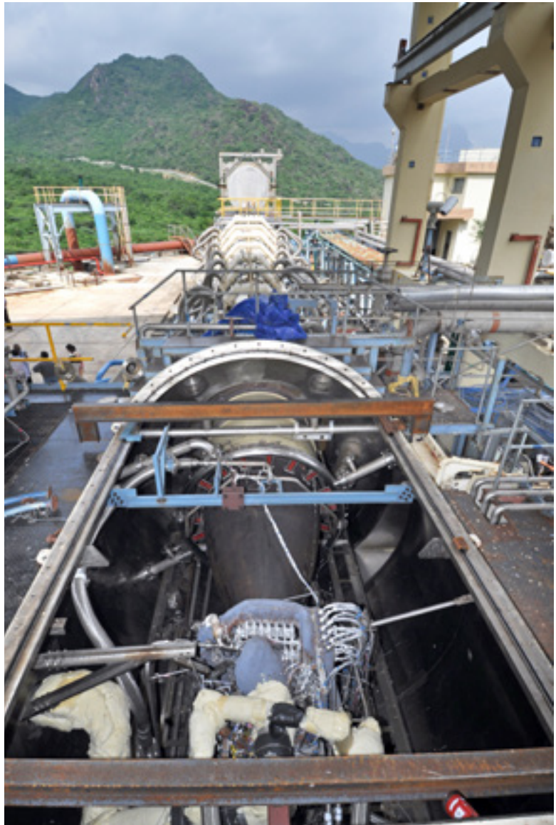
CE20 Engine mounted inside HAT Facility
